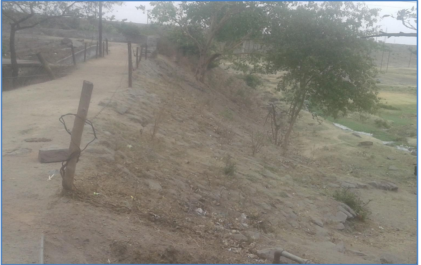
Picture 5 - Stone Pitching/embankment at Kari Jore
