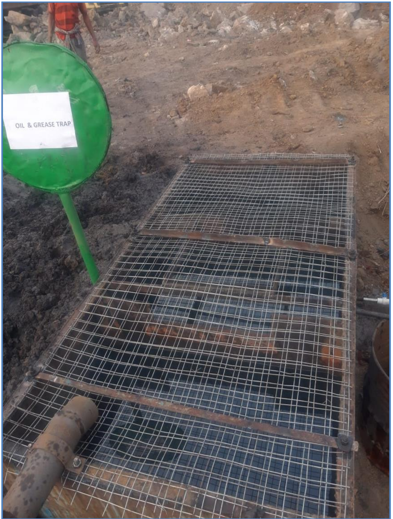
Picture 7 – Oil & Grease Trap
